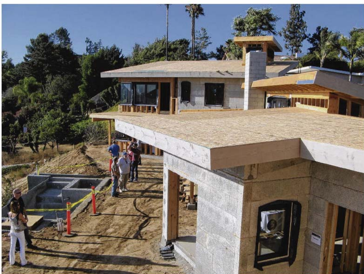
Guests at an architectural reception examine Rhonda and Nigel Farrar's "green home," which is under construction on a spot overlooking Lake Hodges. BRADLEY J. FIKES | bfikes@nctimes.com
