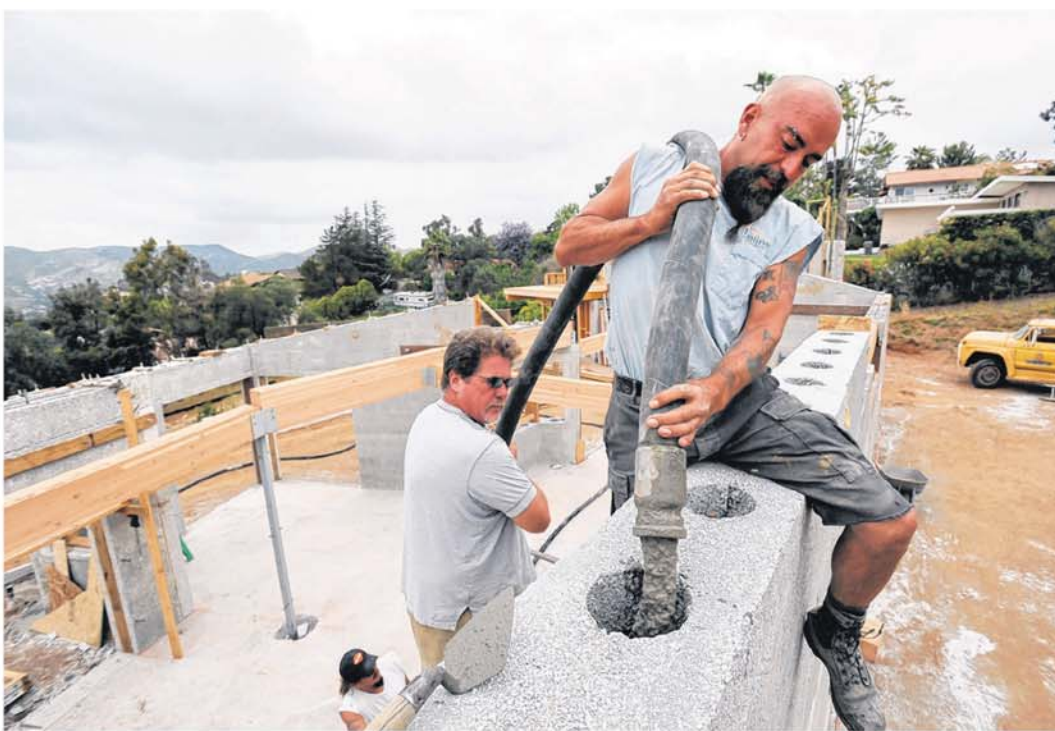
Jerry Gonzales and Pat Lawrence pour concrete into the wall panel system using a line pipe during the construction of an environmentally friendly and energy-efficient home in Escondido.
