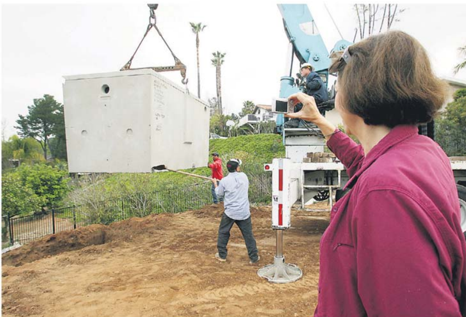
Rhonda Farrar takes pictures Tuesday as a 15,000-gallon septic tank is lowered into the ground at the “green home” that she and her husband, Nigel, are building near Escondido. DON BOOMER | dboomer@nctimes.com
